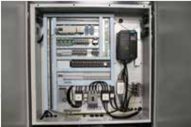
HT & HTS-Electrical System
