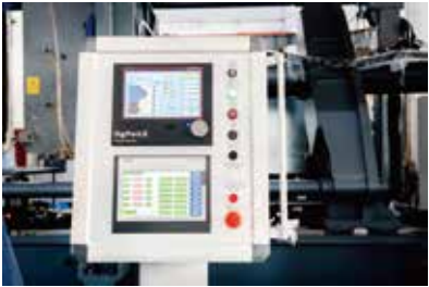
Digital Control System
