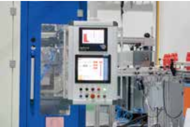
Digital Control System
